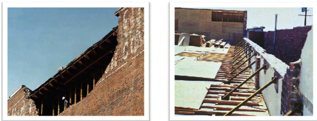
Figure 6.1 Example of parapet failure (l) and parapet bracing (r)
