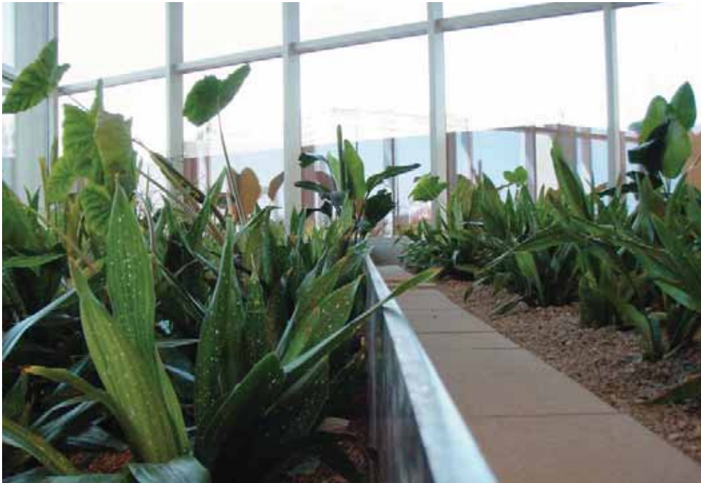
Indoor treatment tanks of the Port of Portland's Living Machine.
