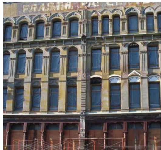
The Bickel Block at 33 NW Couch Street in Old Town is considered by preservationists to be endangered.
